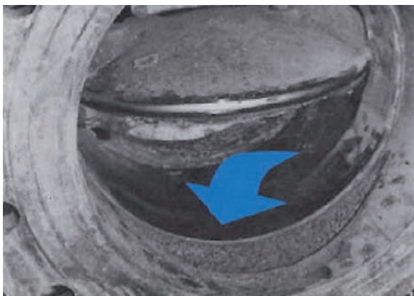
Damage on body
