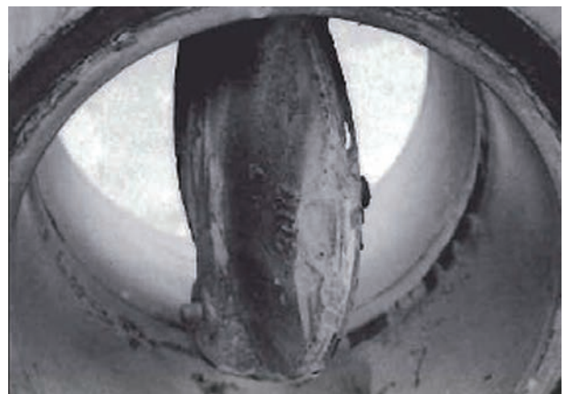
Damage on disc
